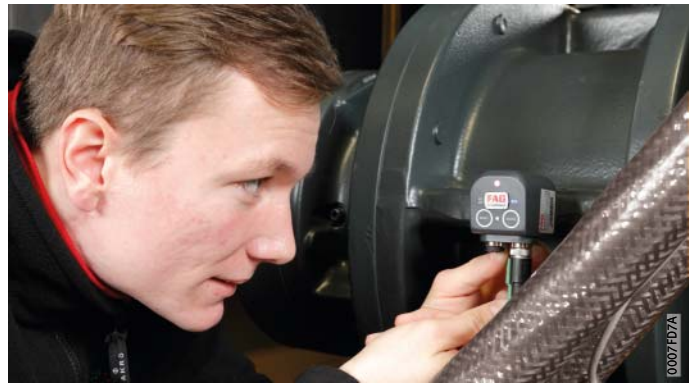
Figure 3 Commissioning of FAG SmartCheck
